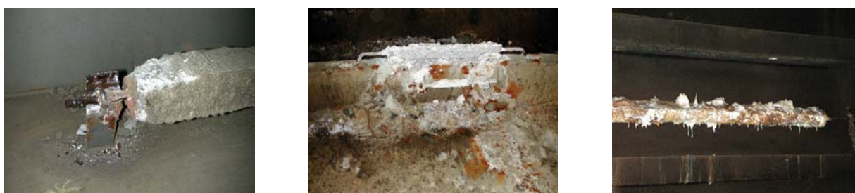
Figure 4-1 Corrosion at Sacrificial Anode; from left to right on attachment only, partially and completely consumed
