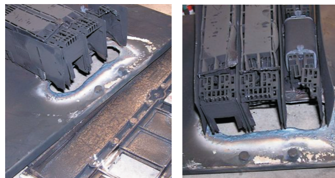
LEFT Arcing fault damage at fault limiters baseplate. RIGHT Another view of the fault limiters baseplate
