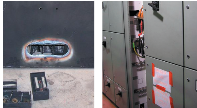
LEFT Rear view of fault limiters baseplate RIGHT The main switchboard cable zone where Michael was working when the incident occurred.
