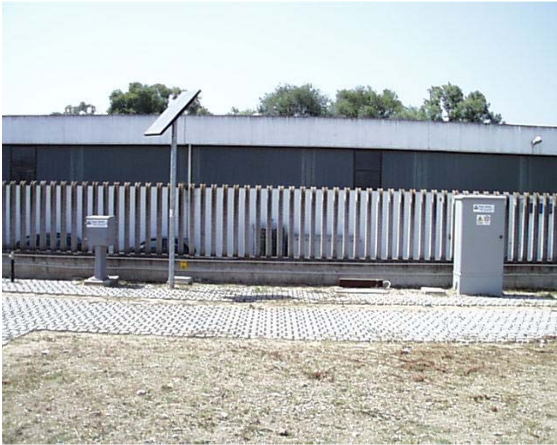
Pic.9 - Photovoltaic installation for cathodic protection and drainage equipment housing
