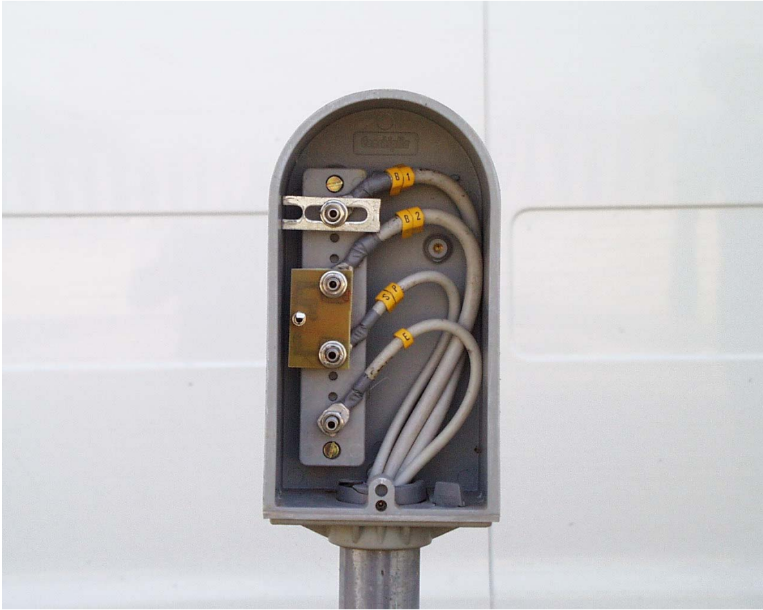
Pic.6 - Permanent test point with terminal board and ON-OFF switch probe
