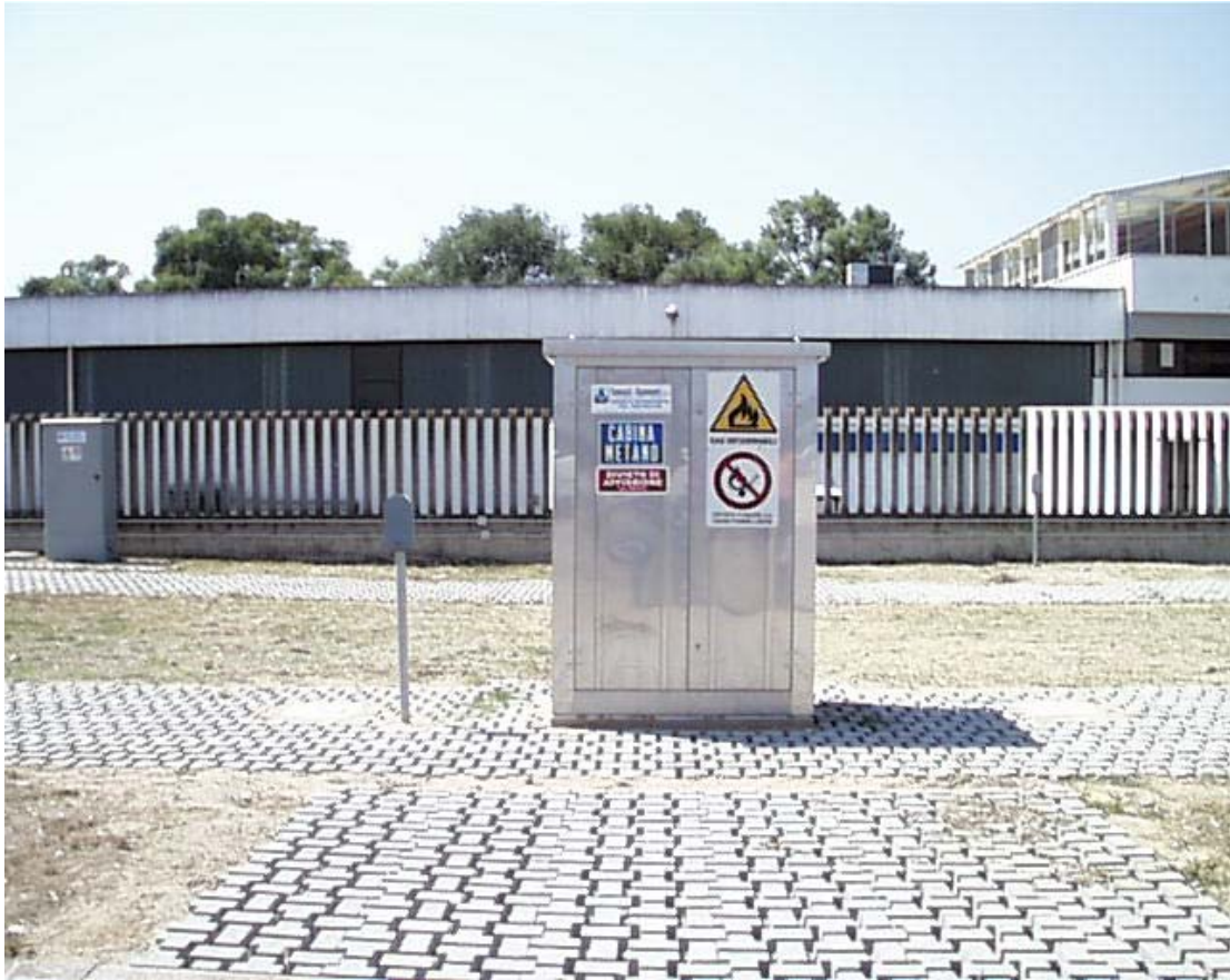
Pic.5 - Final reduction group (GRF) with permanent test point
