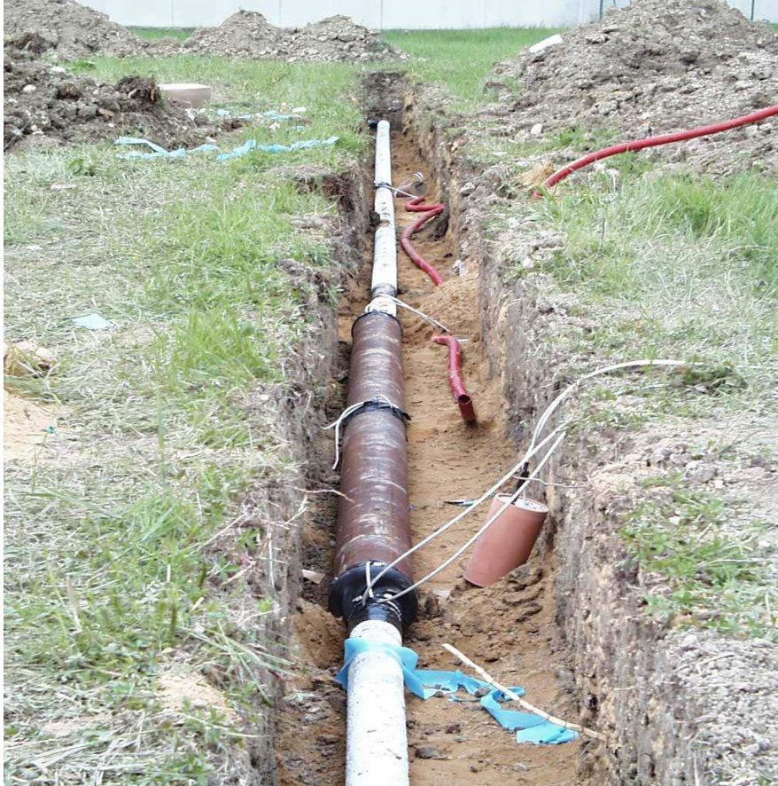
Pic.3 - Railway crossing with cable sleeve
