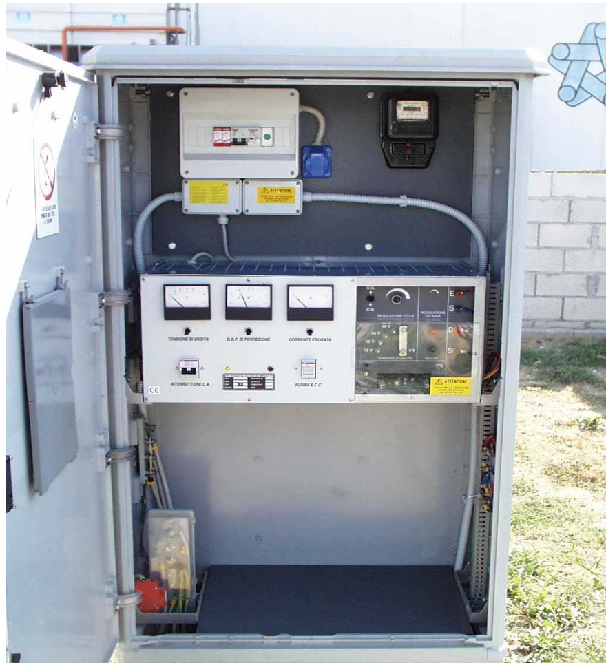
Pic.8 - Typical installation of transformer-rectifier unit with misurament of eletric power meter inside the housing
